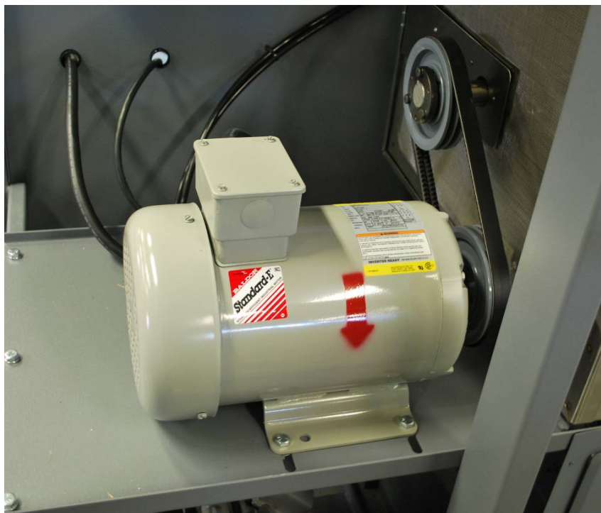
Figure 14 - Main Blower Motor with Direction Indicator
